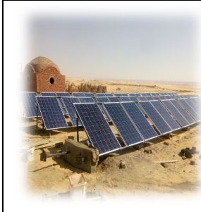
Fig. (25): The Solar System for Water pumping in the new community in the New Valley.
