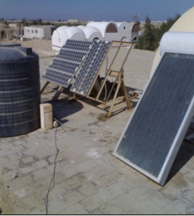
Fig. (21): Overview of the Buildings in the new Community with the solar power units on the roofs.
